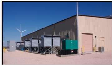
36 MW / 24 MWh Advanced Lead Acid / Li Ion - West Texas
