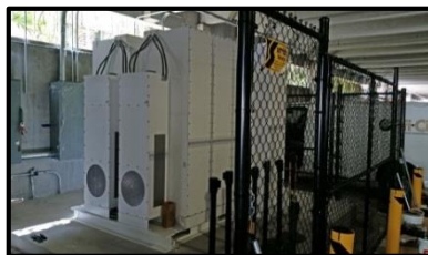
200 kW / 400kWh Lithium Ion - St. Petersburg, FL
