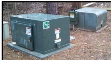
25 kW / 25 kWh Lithium Ion - Charlotte, NC
