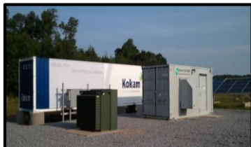
250 kW / 750 kWh Lithium Polymer - Charlotte, NC
