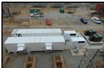
4 MW / 1.5 MWh Beckjord Station - New Richmond, OH
