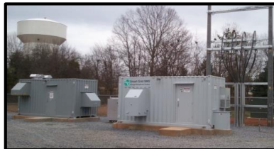
**402 kW / 282 kWh Sodium Nickel Chloride - Mt. Holly, NC
