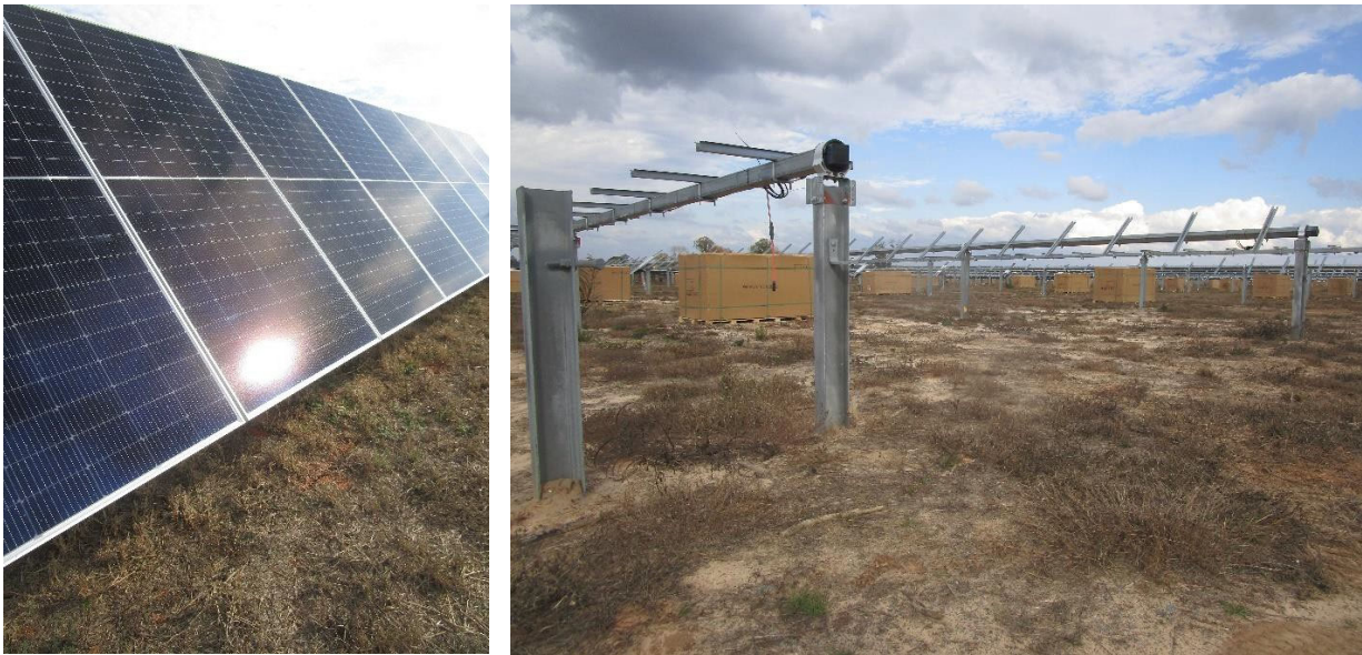
Figure 16-1 — Solar PV Project
