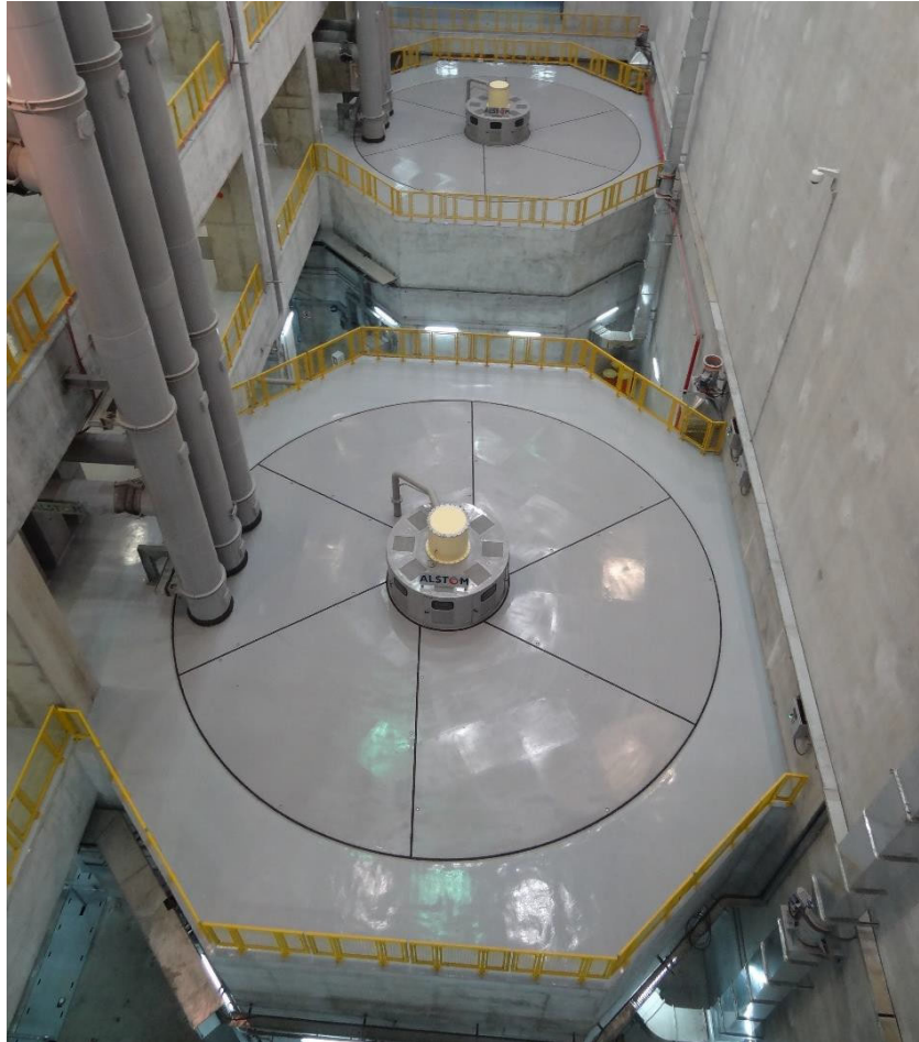
Figure 12-3 — Typical Hydroelectric Power Turbine Hall
